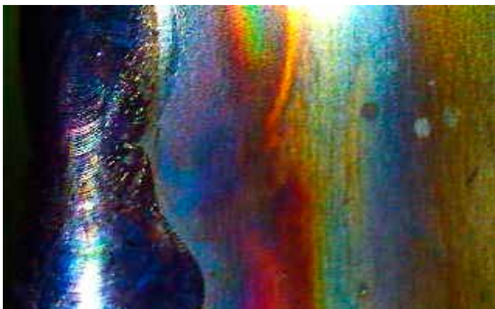
Discoloured heat affected zone on a stainless steel weld. Corrosion protection is severely reduced in this zone.
